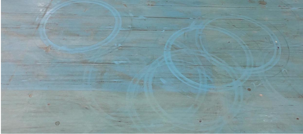
Epoxy Floor - Severe Traces
