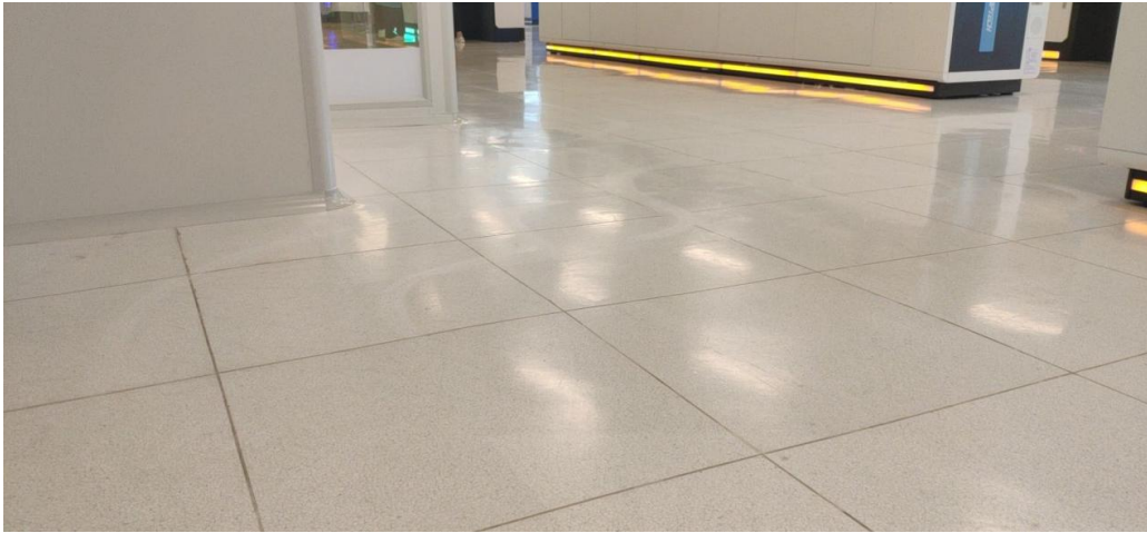
Epoxy Floor - Severe Traces
